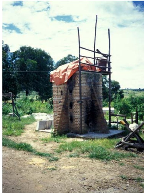
Figure 1: The construction of the experimental kiln, Dedza, Malawi. Photo credit: Practical Action / Kelvin Mason
